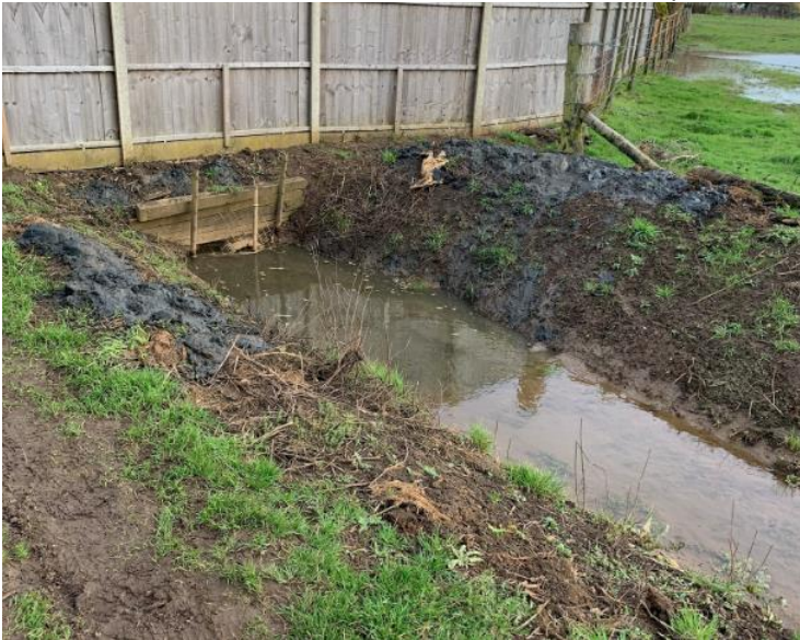
Photos rear of no 7 Orchard Lane 23 Feb – Silt to top of dam sleeper.
