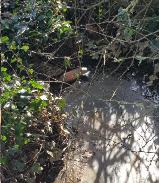
Pipe entry circa 7/8ths silted at inlet.
